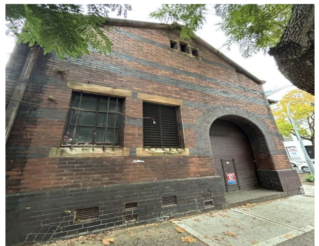
Figure 10 - Southern façade of the electricity Substation showing spalling stone windowsills.
